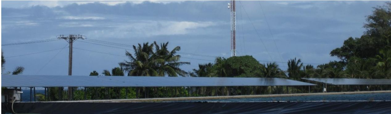
Figure 1.2 – Solar ground mounted PV panels installed around a water reservoir in Majuro atoll
