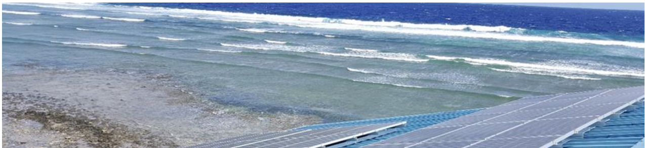
Figure 1.3 - Solar Roof-top mounted PV panels on roof top of College of RMI, Majuro atoll
