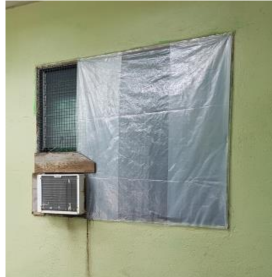
Figure 5: Majuro window style aircon installation, next to window covered in plastic sheet
