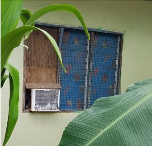
Figure 4: Majuro window style aircon installation, next to louvre windows
