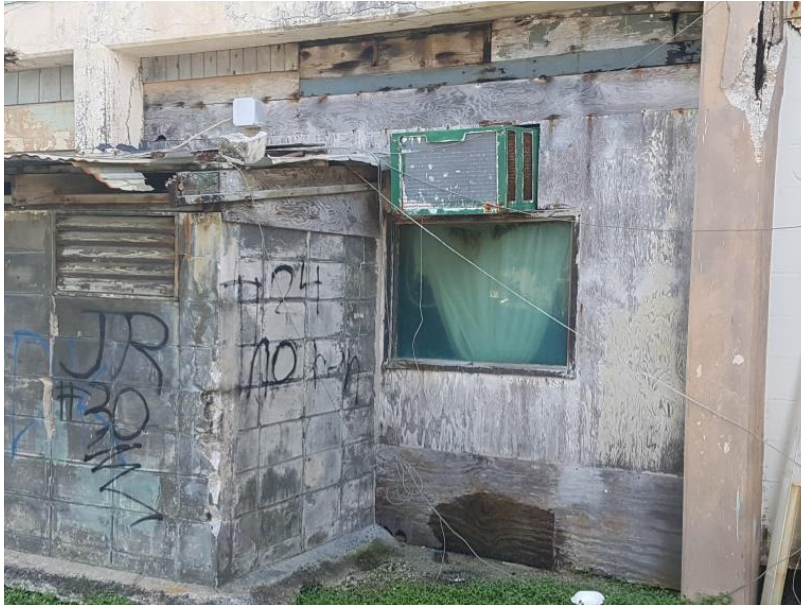
Figure 11 Ebeye air conditioner
